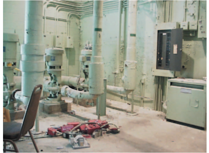
Before/ Equipment Room
