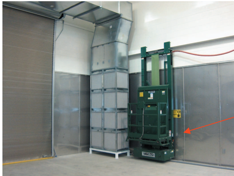
Installed Man Lift
